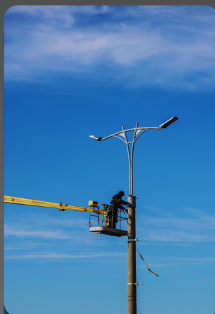
Smart Lamp Pole
